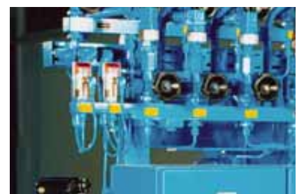
Essential: Temperature monitoring in air conditioning.
